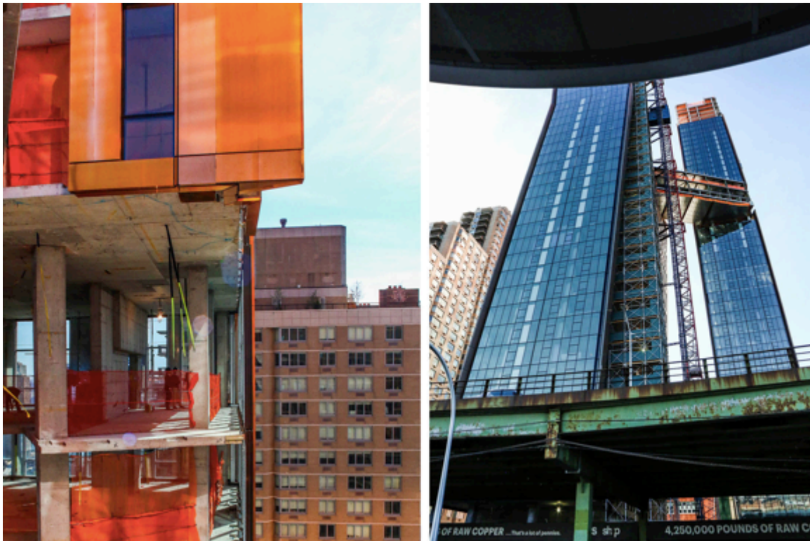
On left: From this vantage point you can see the thickness of the copper cladding. On right: The FDR runs between the buildings and the East River. Photographer: Chris Goodney/Bloomberg
