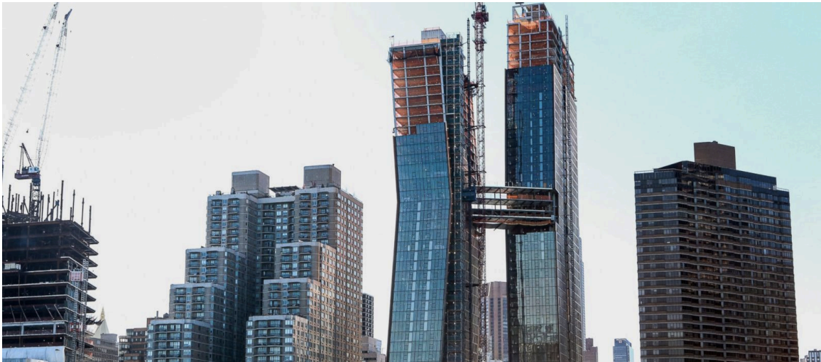
The American Copper Buildings with skybridge stands under construction in New York, April 19, 2016.
