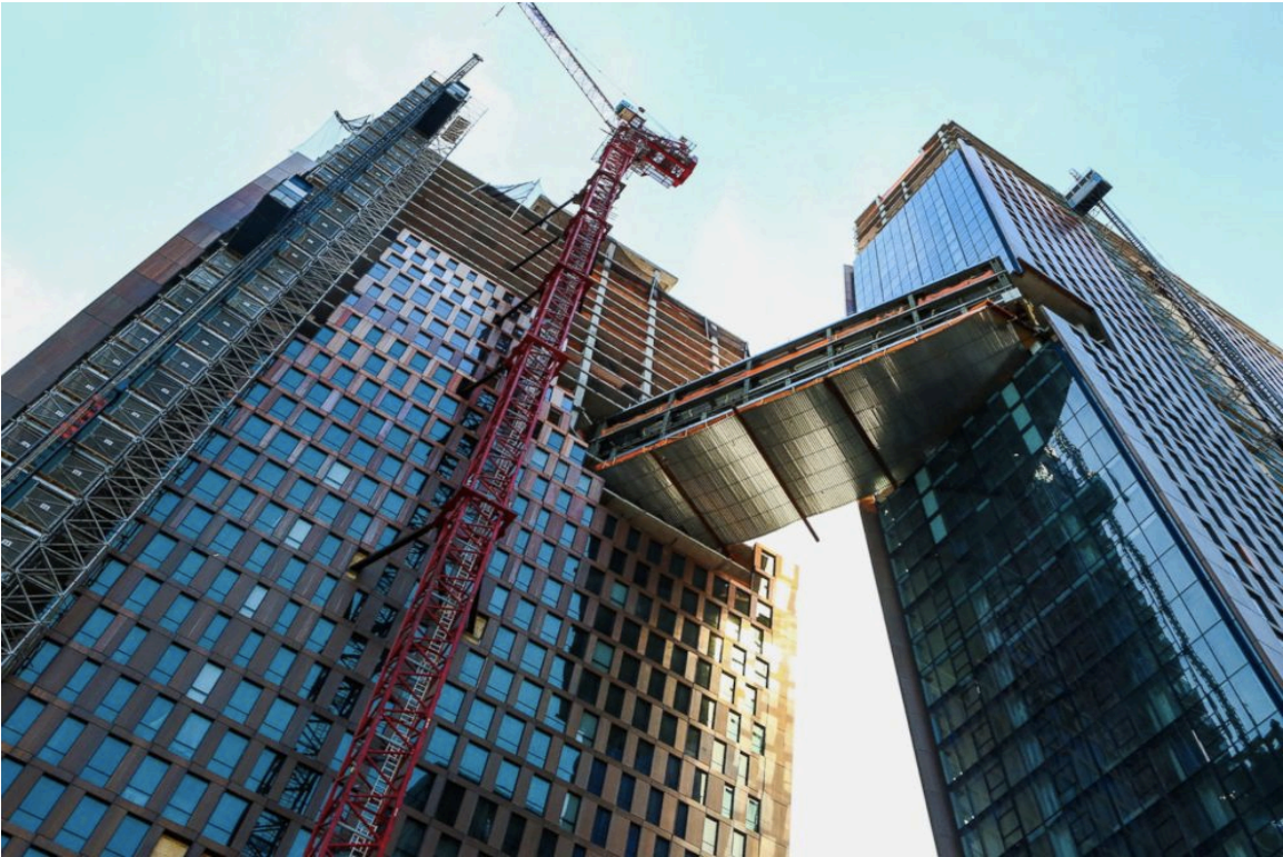
The American Copper Buildings with skybridge stands under construction in New York, April 19, 2016.
